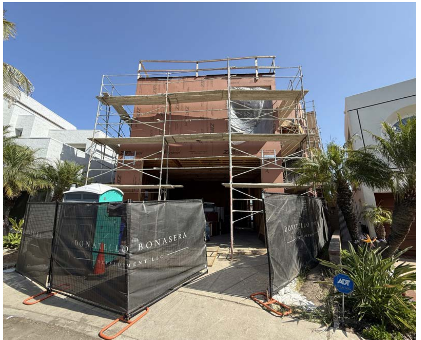
The construction site for the jet house. Donatello Bonasera Development LLC can be seen on the safety netting. Staff photos by Madeline Yang.
