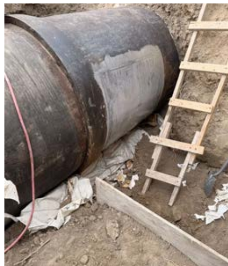
A leak in the Parallel Gravity Line began emergency repairs on May 14, which were completed on May 16. Photo by IBWC.
