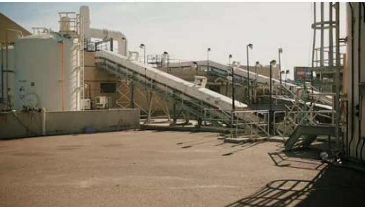
FILE: The South Bay International Wastewater Treatment Plant, pictured here, now can process 10 more mgd of sewage. Staff photo by Madeline Yang.
