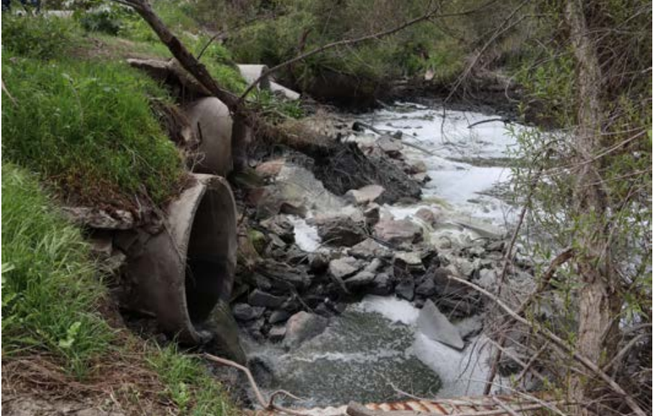
Scientists say culverts, the tunnel-like pipes transporting wastewater below Saturn Boulevard, cause high turbulence that exacerbates water-to-air transfer of toxic wastewater pollutants in the Tijuana River. Staff photo by Julieta Soto.
