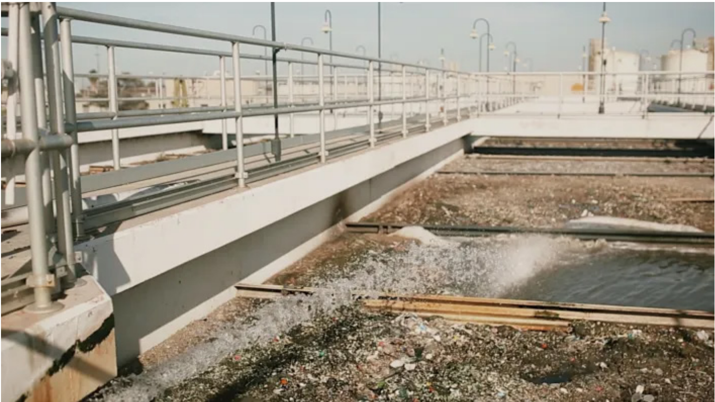
This primary sediment tank at the South Bay International Wastewater Treatment Plant, which is operated by Veolia North America, is overloaded with trash. The role of the tank is to remove solids from the wastewater. Staff photo by Madeline Yang.
